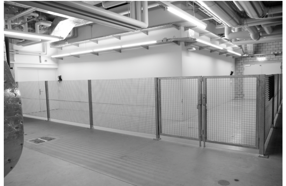
From the view of the projector Technical room, basement HSLU K&D, Viscosistatt
